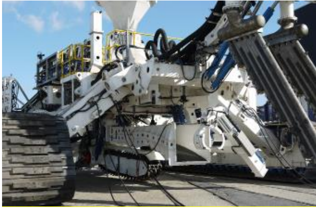
Plate 3 - The trench created during mechanical trenching can be back filled or left to refill through natural sedimentation.
